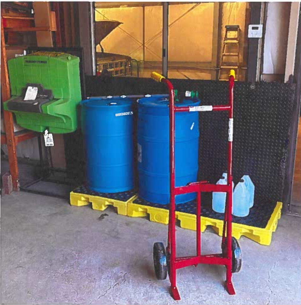
Added Chlorine spill containment for 50 gallon bulk deliveries.
