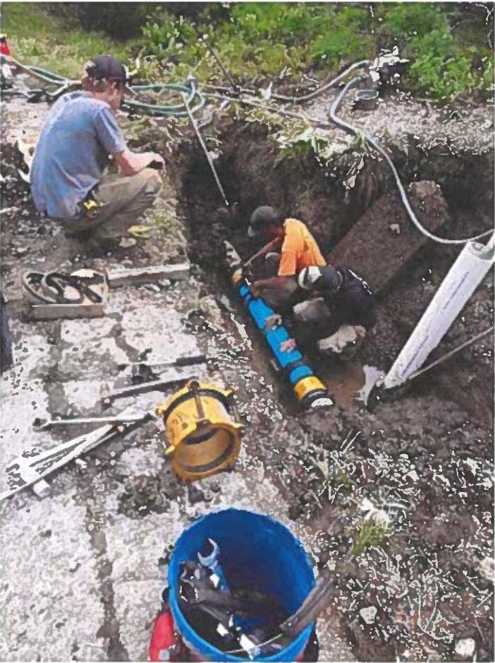
May 21 st water leak at the ski resort subway parking lot access road just down from the Achieve Tahoe building
